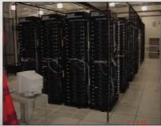
Google data Center (2008)
